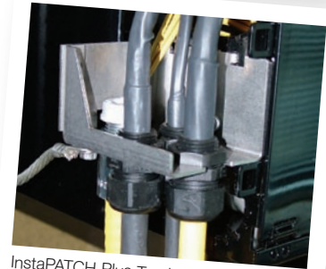
InstaPATCH Plus Trunk Cables attached to shelf mounted bracket
