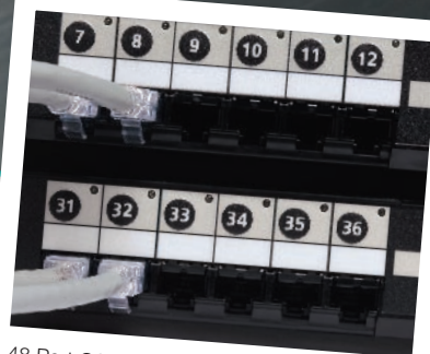
48 Port GS3 – close up
