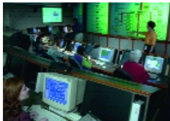
At its Data Services Center in Tampa Bay, Fla., Avaya monitors and maintains 10,000 enterprise servers and switches for customers across the United States.
